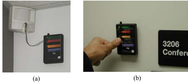
Figure 6: Conference room (a) motion sensor node and (b) reservation status indicator.
