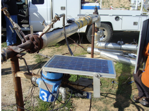
Figure 16: Invasive flow sensing with solar panel for power.
